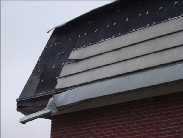
Falling and missing fascia and siding on vacant service station.
