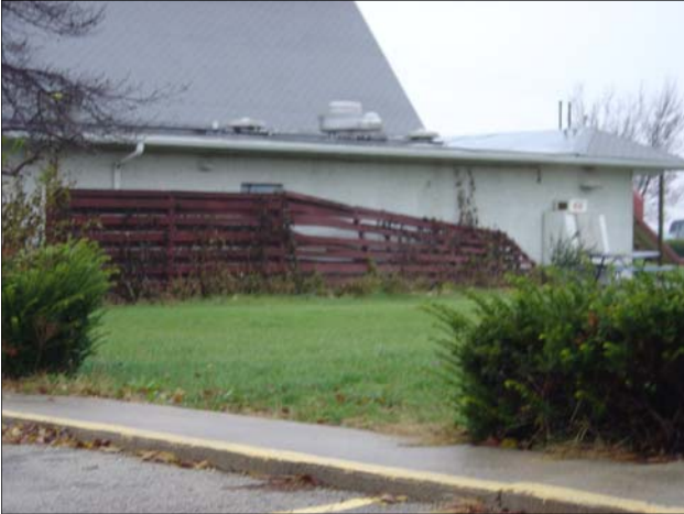
Deteriorated fence on Budget Inn.
