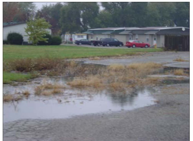
Standing water on deteriorated parking lot in rear of vacant hotel.
