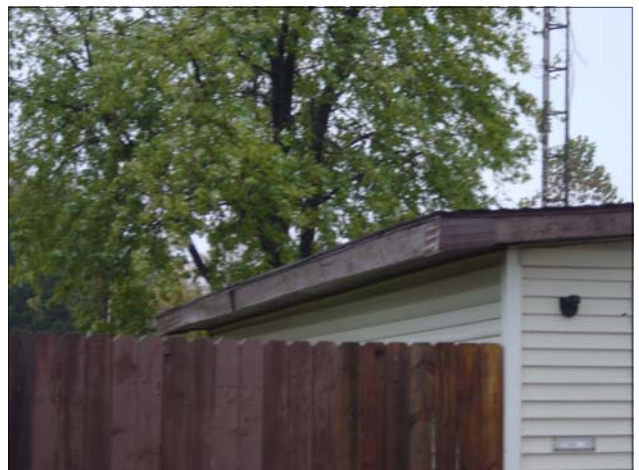
Deteriorated fascia on front of residence.
