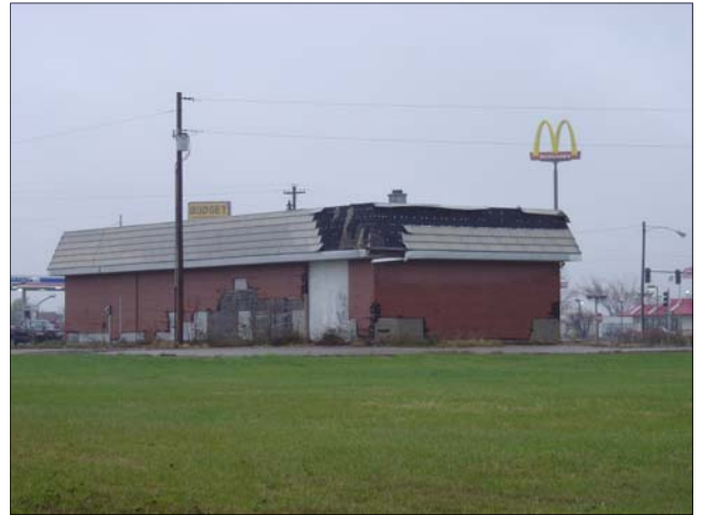
Deteriorated vacant service station at the southwest corner of Paradise Road and South Route 45.
