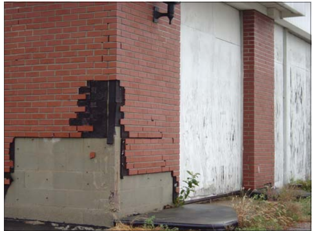
Falling and missing brick siding on vacant service station. Note boarded doors.
