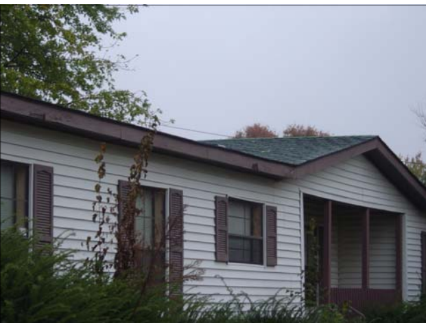
Deteriorated fascia on front of residence.
