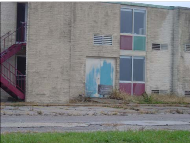
Deteriorated door and parking lot of vacant hotel
