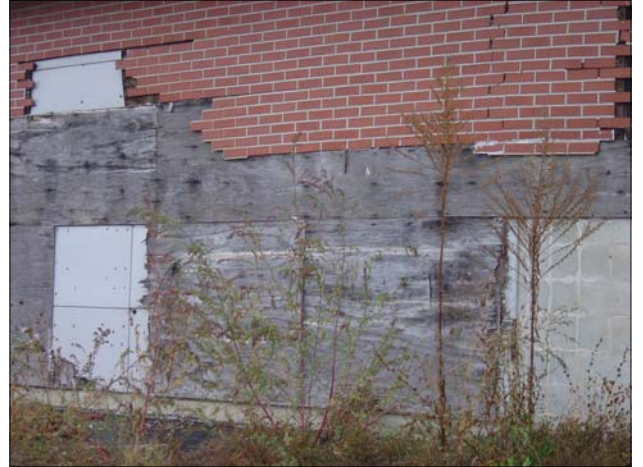
Falling and missing brick siding on vacant service station.
