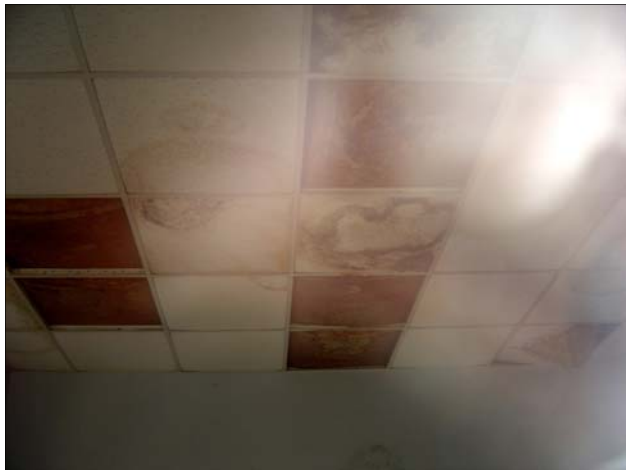
Water damage on ceiling tiles in vacant hotel.
