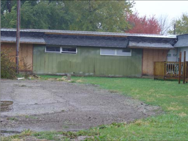
Dilapidated two-family apartment building with deteriorated siding and boarded windows.
