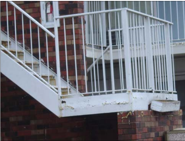
Peeling paint and rusting stairs on Budget Inn.
