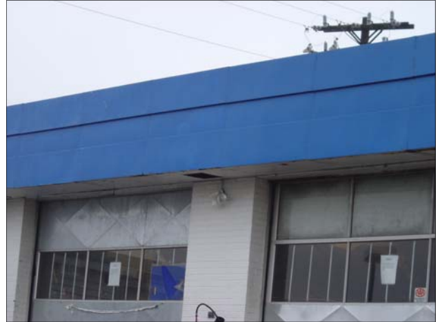
Broken window and damaged soffit on Marathon Service Station building at northwest corner of Paradise Road and South Route 45.
