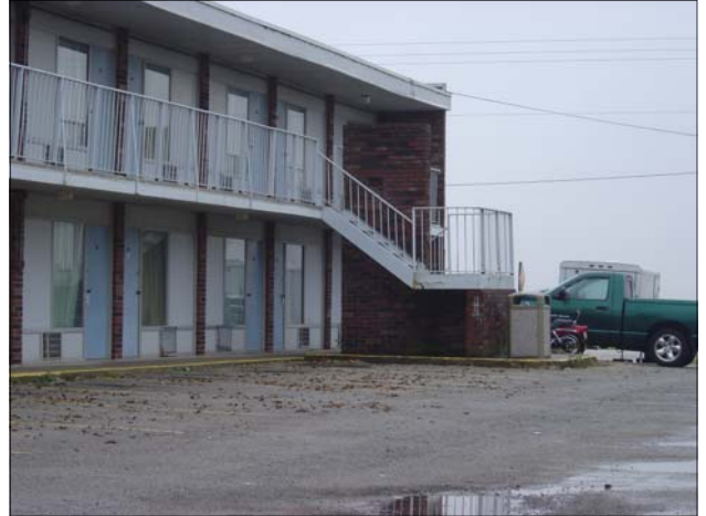
Deteriorated stairs and parking lot of Budget Inn.
