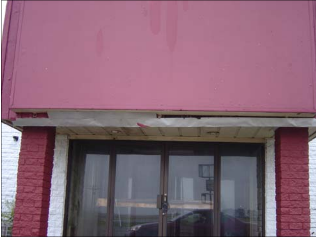
Deteriorated fascia on front entrance of vacant hotel.
