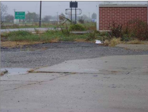
Deteriorated parking lot of vacant service station
