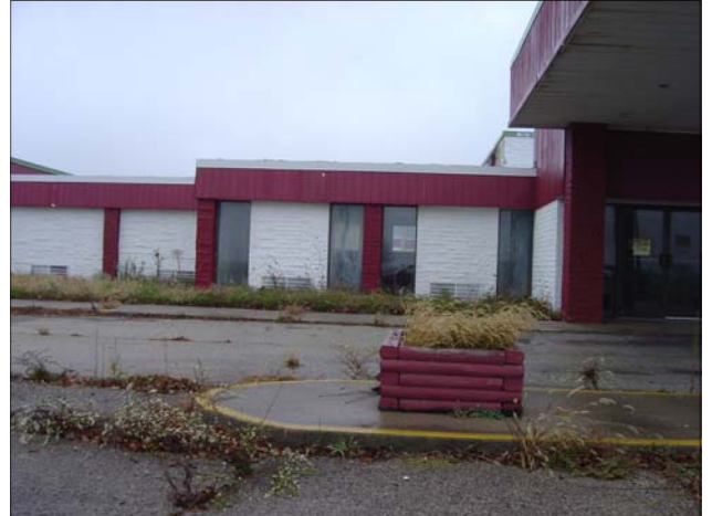
Deteriorated parking lot of vacant hotel.
