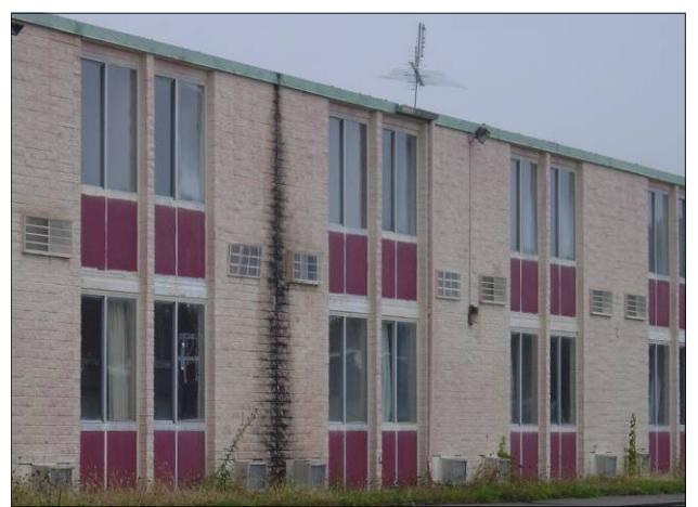
Rear of vacant hotel. Note water damage on bricks and mortar.
