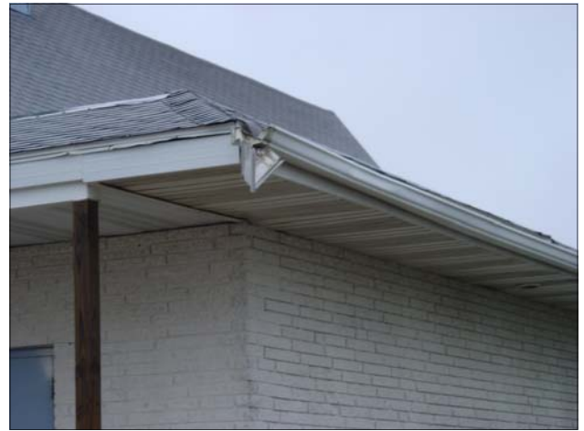
Damaged gutter on Budget Inn building.
