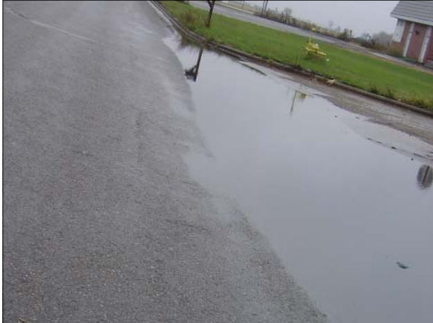
Standing water on south side of Paradise Road.
