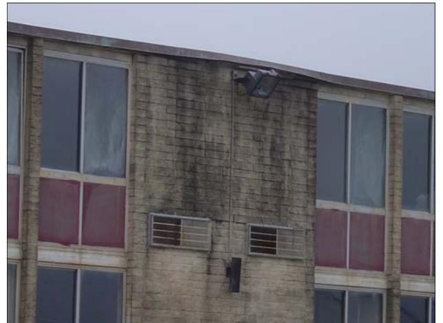
Rear of vacant hotel with deteriorated bricks and mortar.
