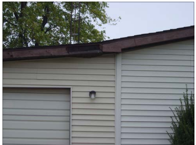
Deteriorated fascia on residence on Carter Lane.
