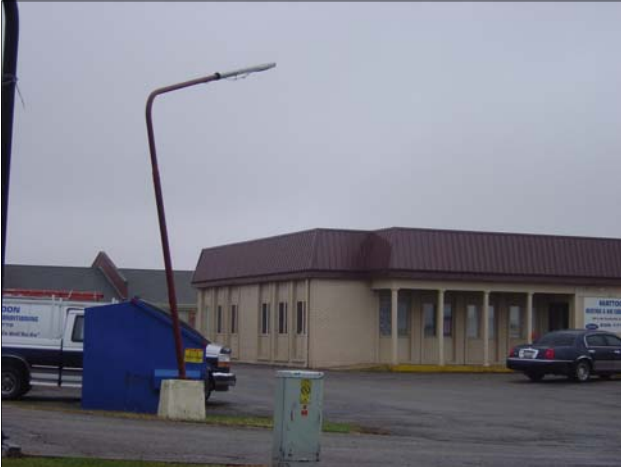
Broken and leaning light on Mattoon Heating and Air Conditioning parking lot. Note deteriorated parking lot pavement.
